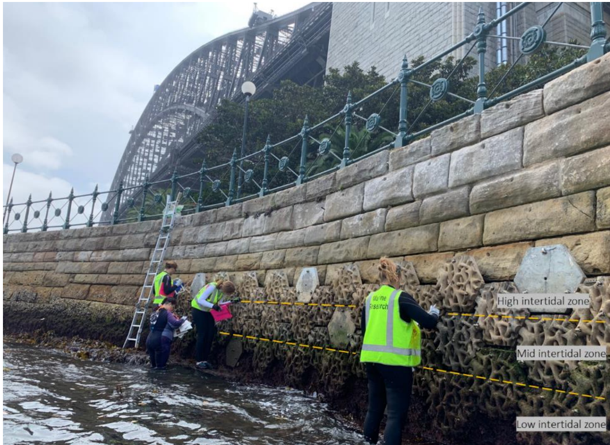
Figure 2: Volvo Living Seawall installation along the Bradfield Park seawall in Milsons Point, New South Wales, Australia. Intertidal biodiversity was sampled in the high, mid and low intertidal zones. Image credit: Maria Vozzo, SIMS.
